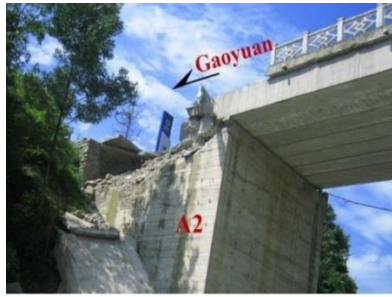
(b) The damage of A2 abutment
