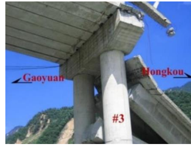
(c) The slippage of girders
