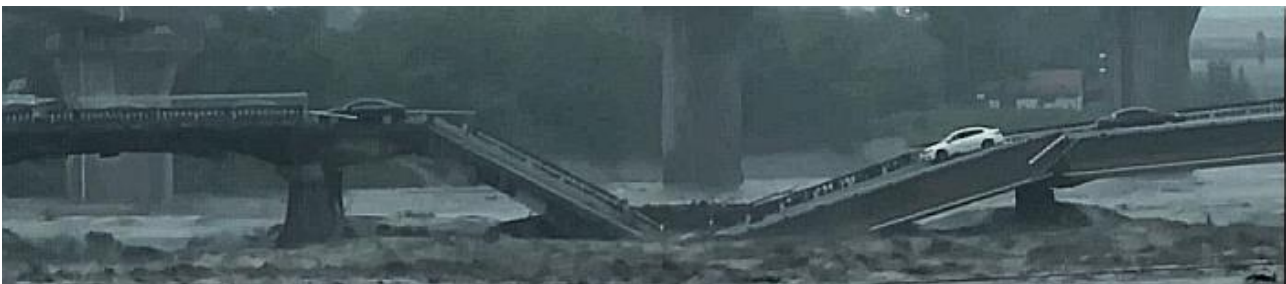
Figure 5. Xiaoqing River Bridge Field pictures of the fracture point [6]
