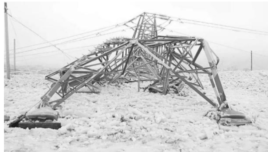
Figure 1 Power transmission tower collapsed by snow and ice disaster
