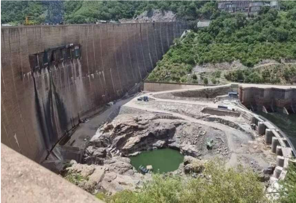
Figure 2. Extreme heat impact on the Kariba Dam as main hydro-power station in zambia
