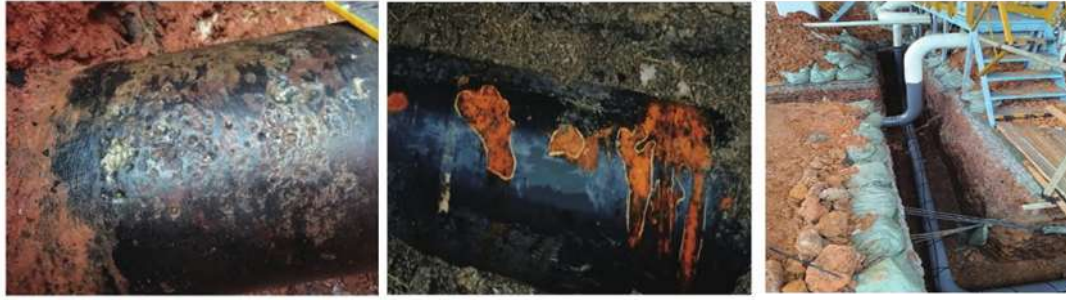
Fig. 1 Exterior View of Corroded Buried Pipelines in an Oil Transfer Station
