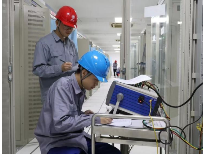
Figure 2. Ultra-high voltage substation relay protection equipment
