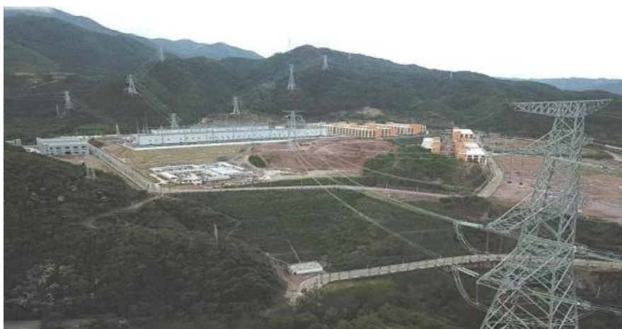
Figure 1. Ultra-high voltage substation
