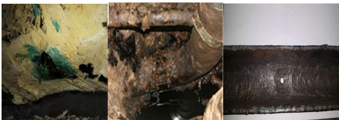
Figure 1. Corrosion perforation pictures
