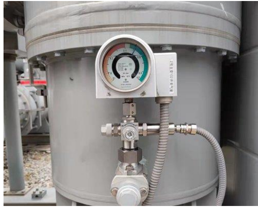
Figure 2.9. Gas detection of GIS equipment
