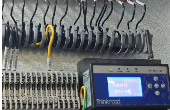
Figure 2.13. Wireless temperature measuring terminal in switchgear
